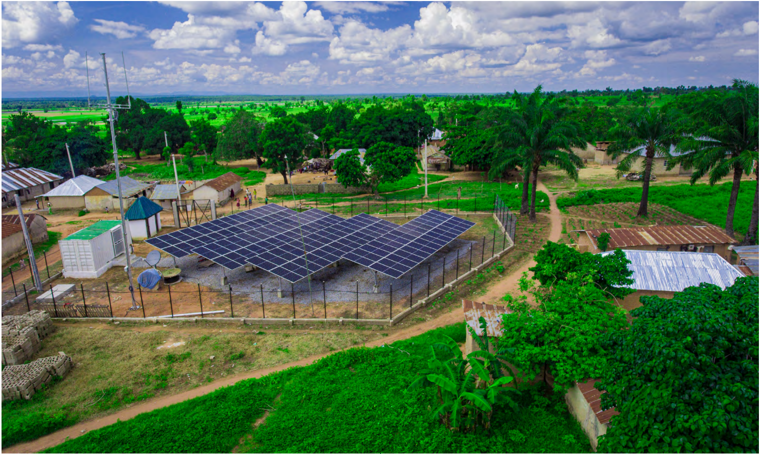
Husk non-interconnected mini grid in Akura community, Nasarawa State, Nigeria.
